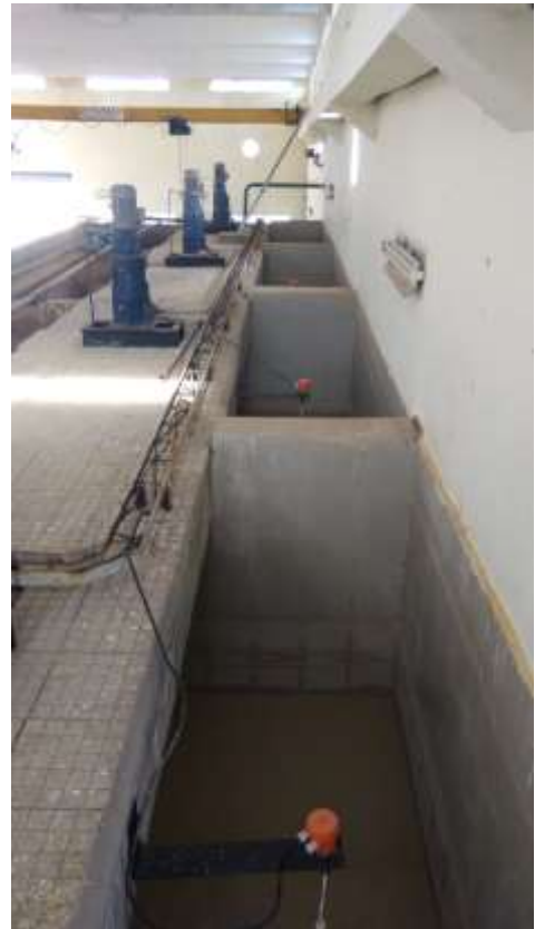
ALUM TANK LEVEL MONITORING
